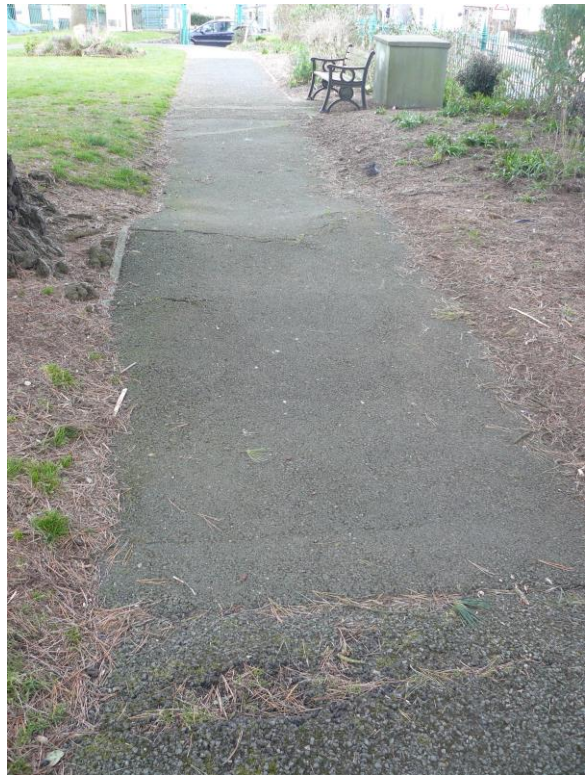
displaced tarmac adjacent to fir tree
