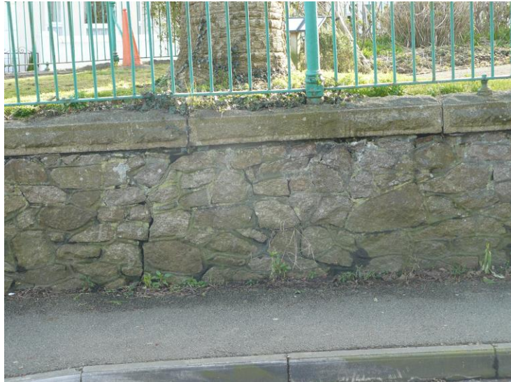
displaced masonry adjacent to Araucaria Araucana tree
