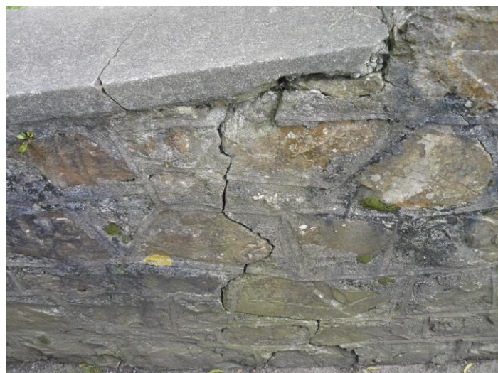
settlement of wall adjacent to higher Callington Road entrance
