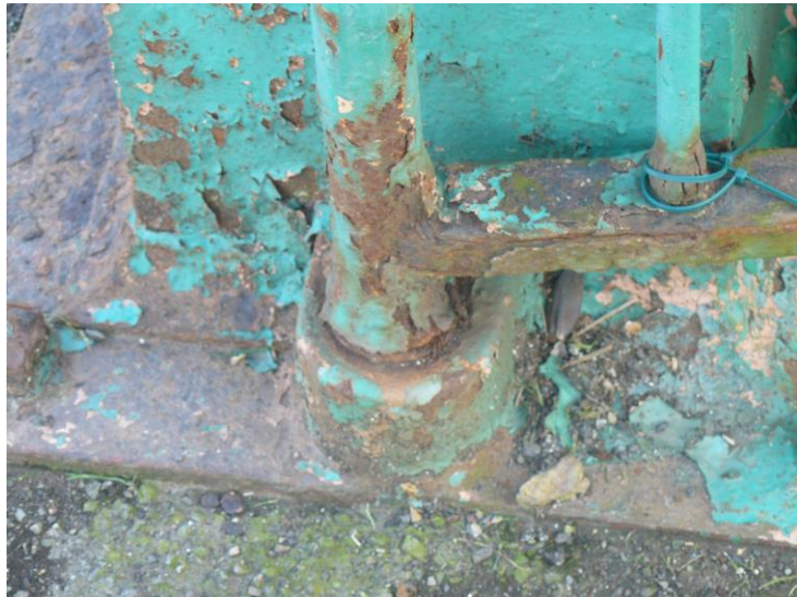
corrosion to east gate
