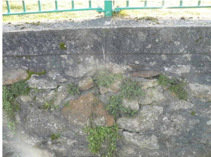
example of weed growth & defective pointing
